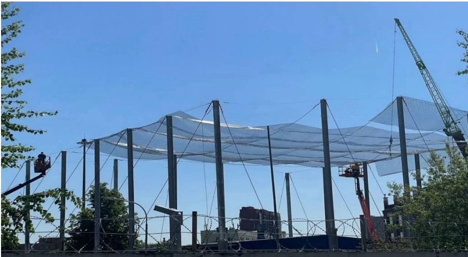
Figure-3: Netting to protect critical systems
