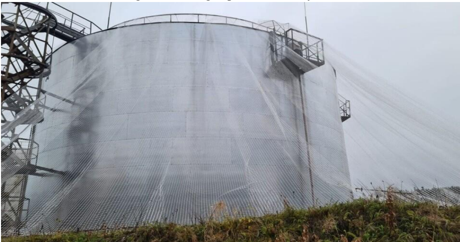
Figure-4: Netting to protect fuel storage tank.
