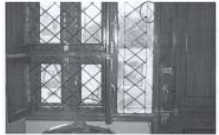
Two example of strengthening of grill by welding V-shaped metallic strips over the nails. Also note that the door is too close to the window and the house owner is forced to lock the door from inside to avoid its opening through the window
